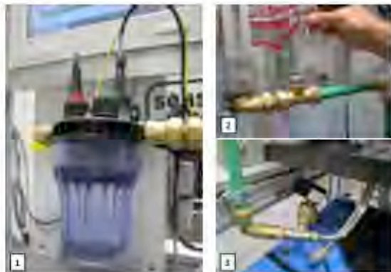
Figure 1. Probes: temperature, chlorine, conductivity and pH. Figure 2. Temperature probe: upstream of the shower and the sink. Figure 3. Electrovalve
